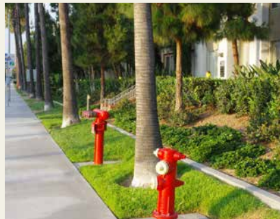
Fire hydrants installed outside the pedestrian through-zone. Jamboree Road, Irvine
