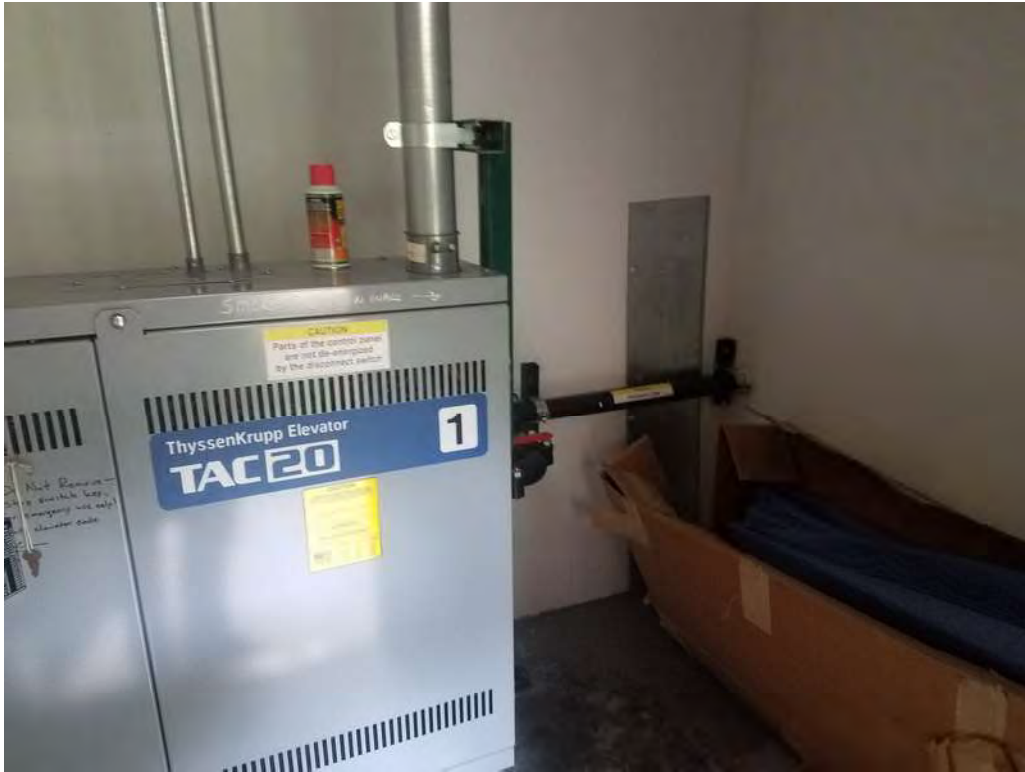
View of elevator equipment in 23591 building.
