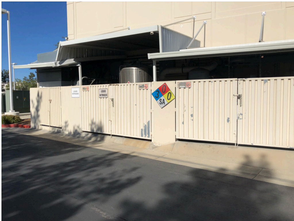
Location of large liquid nitrogen AST on east side of building, facing west.
