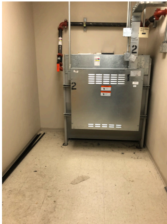
Typical elevator equipment room.
