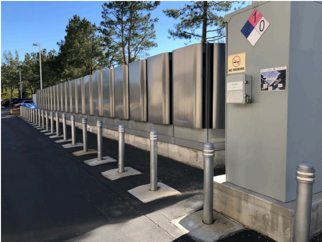
Fuel cells along eastern property boundary, facing northeast.
