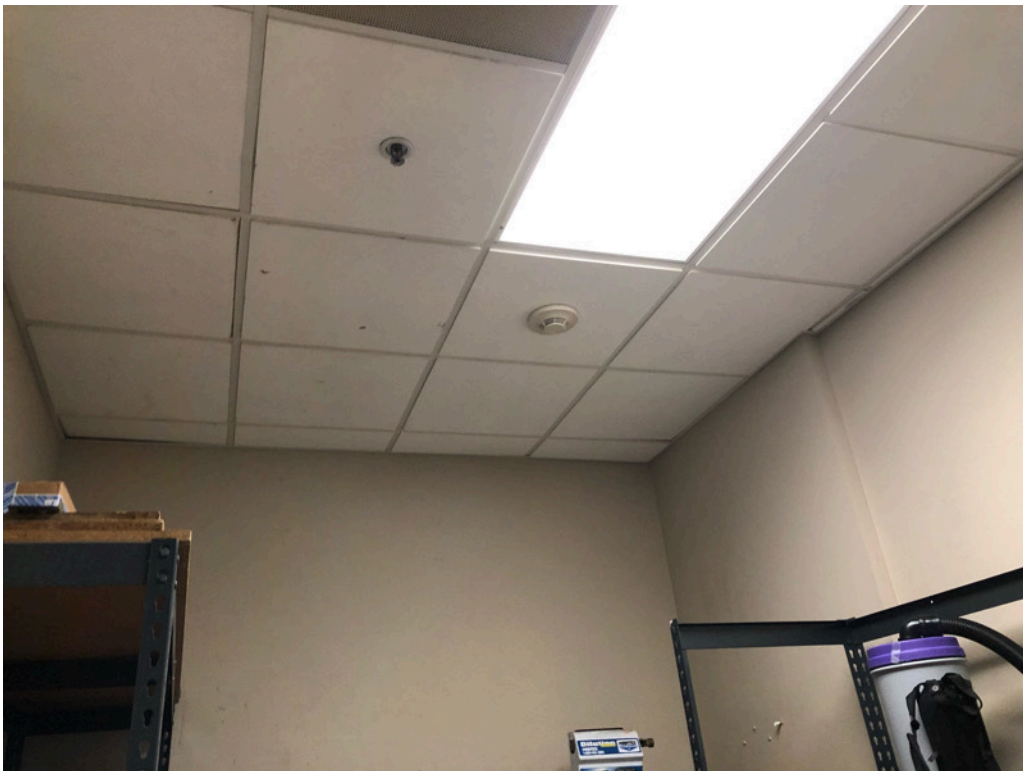
Typical acoustical ceiling panels.
