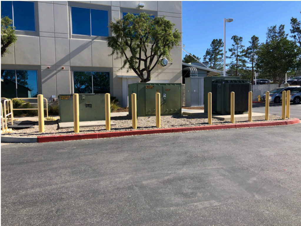
Pad-mounted transformers located at southeast corner of building, facing north.
