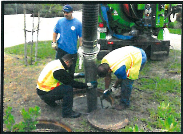
Insert Vacuum Hose to Remove Trash & Debris from the Screening Basket.
