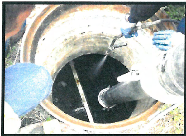
If Sediments are Compacted Use a Pressure Washer to Loosen Up Sediments.
